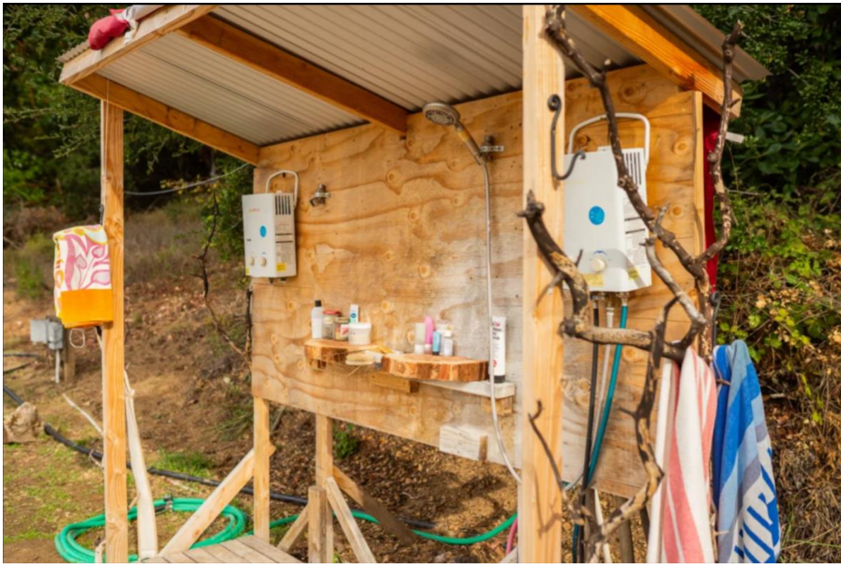
Figure 8b. Outdoor shower with propane heaters and electrical conduit on the ground. The propane heater at the right is suspended loosely by a single nail.
